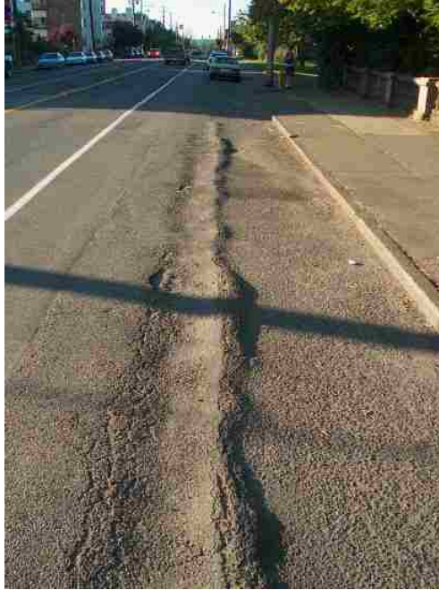
Figure 2.1 Permanent deformation distress
