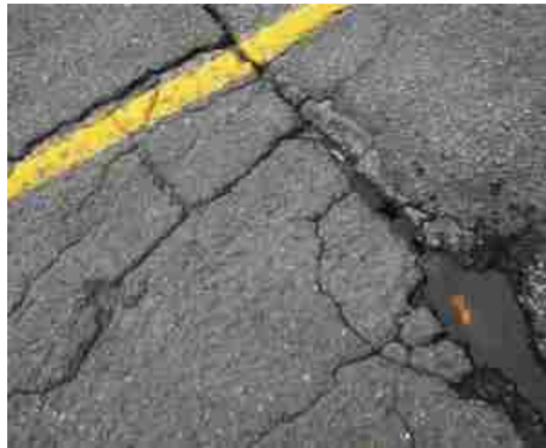
Figure 2.3 Moisture damage in asphalt concrete
